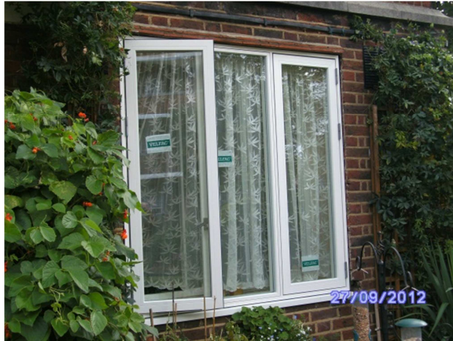
New sample window (aluminium clad timber double glazed) to the right hand lower ground floor flat.
